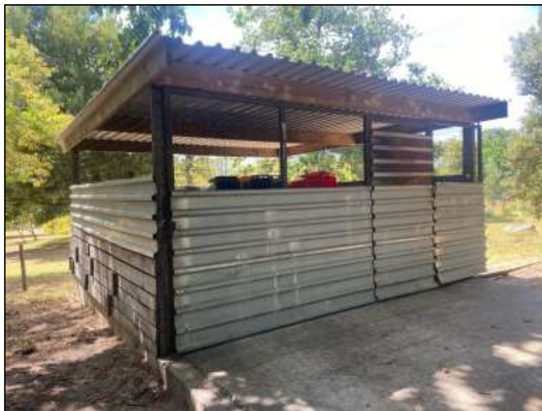
Figure 2. Well-secured waste at Chrysalis Academy.
