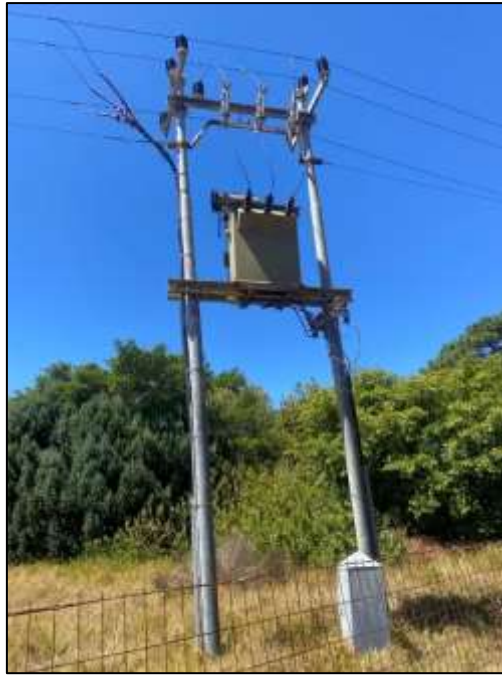
Figure 7. Part of the electricity line at Berg Farm which has been highlighted for mitigation.
